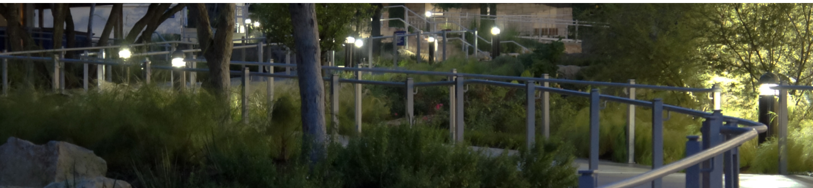
Pictured Below: Riverbend Church's existing walkway bollard lights were retrofitted with ActiveLED ® components saving 83% in energy.
